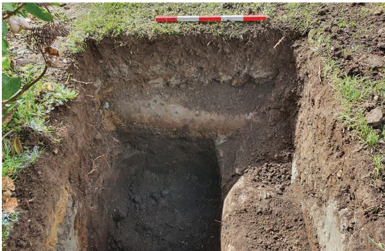
Figure 7. View east of insertion hole outside 2 Ritimona Street showing 300 mm stormwater pipe.
